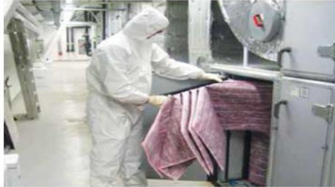
Figure 9: Personal protection equipment for filter replacement
